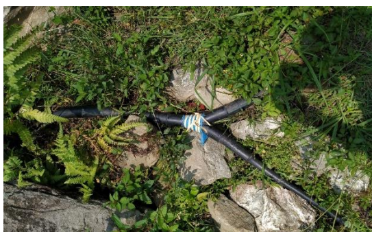
Fig. 17: Exposed HDPE pipe and the tee at Simle Badahare Muhan Ghari Guru Gaon W/S Scheme, Bhorle, Rasuwa (HDPE pipe should be kept at 3 feet and the tee should be kept in a distribution chamber equipped with gate valves to control the discharge)
