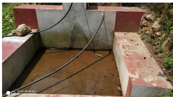
Fig. 18: HDPE pipes connected to the taps and flooded platform at Simle Badahare Muhan Ghari Guru Gaon W/S Scheme, Bhorle, Rasuwa (Unfinished floor and wall of the chamber and the tee of the outlet pipe is redundant)
