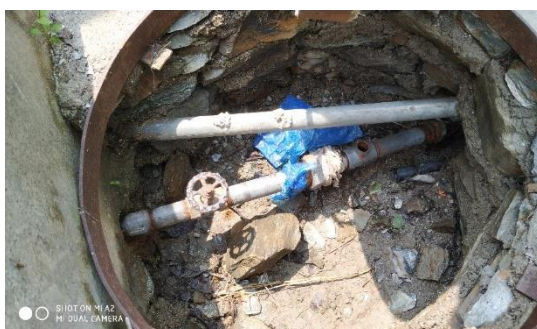
Fig. 15: Poorly constructed valve chamber at Simle Badahare Muhan Ghari Guru Gaon W/S Scheme, Bhorle, Rasuwa (Unfinished floor and wall of the chamber and the tee of the outlet pipe is redundant)
