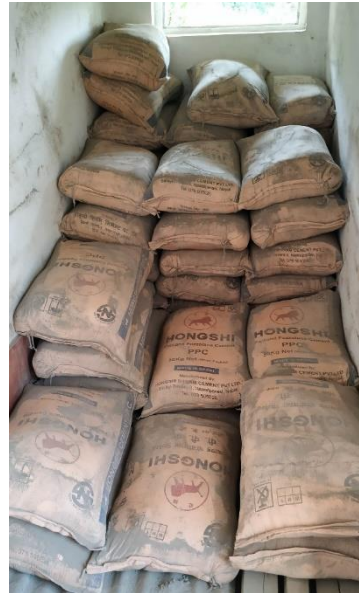
Fig. 4: Girls urinal room in Nuchet Primary School, Nuchet, Bhalche being used to store cement, The toilet was constructed under American Red Cross and Spanish Red Cross
