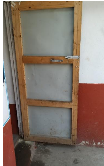
Fig. 8: Position of inside lock in the toilet of Nuchet Primary School, Nuchet, Bhalche, The toilet was constructed under American Red Cross and Spanish Red cross
