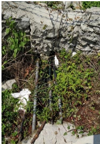
Fig. 9: Water collection pipes at the downstream side of Heping W/S Scheme (Valve Chamber was not constructed, as of this the maintenance works would be difficult)
