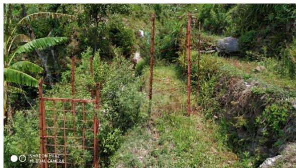
Fig. 16: Poorly constructed fencing and the entrance at Simle Badahare Muhan Ghari Guru Gaon W/S Scheme, Bhorle, Rasuwa (Strangers and the animal can enter the intake premises and error on the entrance)
