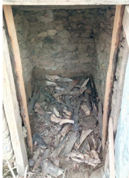
Fig. 22: A Latrine in one of the beneficiaries of Pakani Thada Khola W/S Scheme, Gogane - 8, Makawanpur (It is used to keep firewood.)
