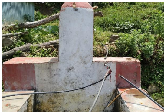
Fig. 3: HDPE pipes (6 in nos.) used for getting water directly at the individual houses compromising the objective of public tap stand post, this is also the potential source of conflict (Heping W/S Project, Bhalche, Nuwakot)
