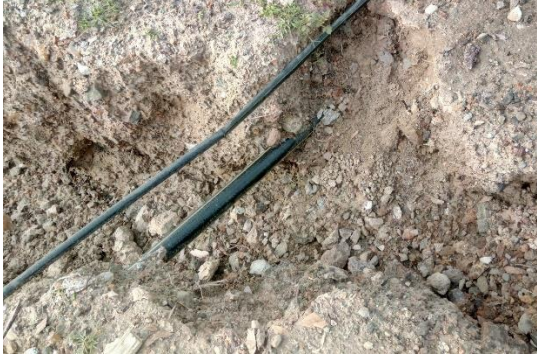
Fig. 21: Exposed HDPE pipes at Jantare Khola W/S scheme, Thaha -5, Makawanpur
