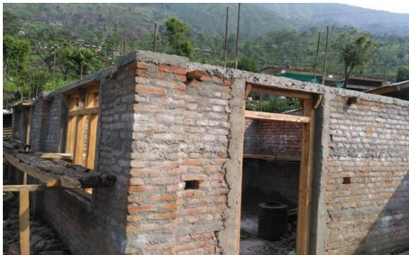
Fig. 2: An incomplete house in Rasuwa. Construction stopped 6 months ago, but the owner still received all the grant instalments.
