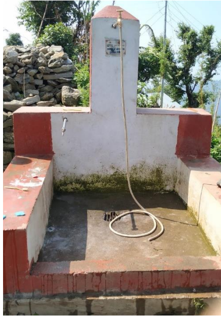
Fig. 1: Plugged lower tap meant for children (Heping W/S Project, Bhalche, Nuwakot)
