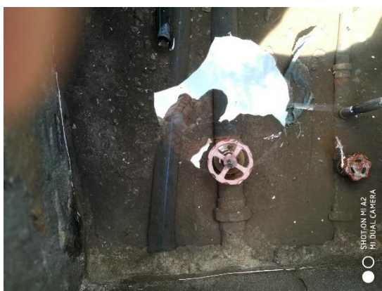
Fig. 19: Valve chamber at the intake of Sisneri Muhan Ghari Gumbadanda W/S Scheme, Bhorle, Rasuwa (Gate valve and the pipes are under water as of the leaking wall, an equal amount of tapped discharge is wasted on the intake periphery as of faulty design, VMW said that he could not mobilise the UCs to repair these )
