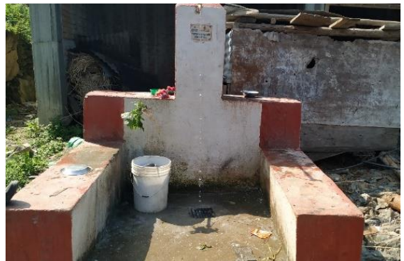
Fig. 2: Lower tap plugged by stinging nettle plant to avoid children reach (Heping W/S Project, Bhalche, Nuwakot)
