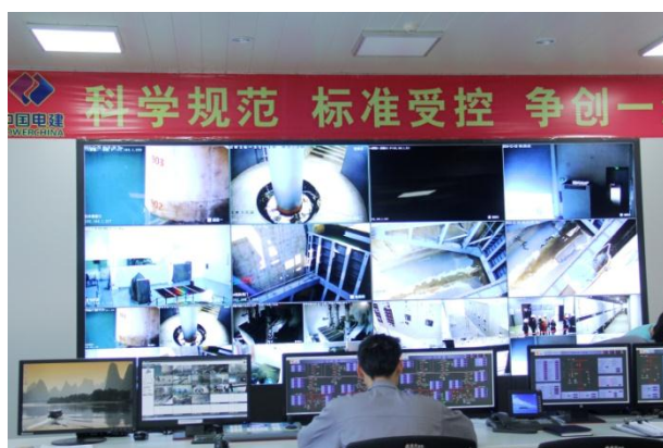
Control room of Upper-Marsyangdi A HEP
