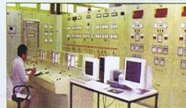
Power House Control Room
