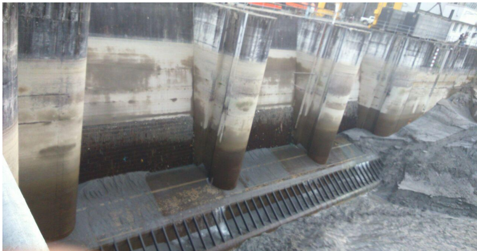
Figure 2-8: Deposition of sediment in and around intake trash rack (Source: NEA , 2016 b)
