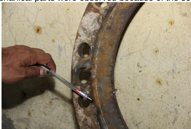
Figure 2-6: Erosion in electro-mechanical part
