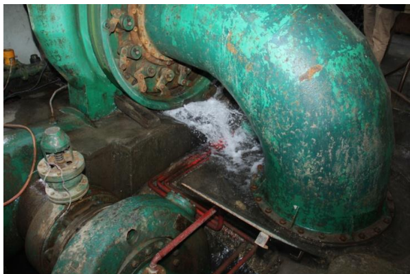
Figure 2-5: Leak in turbine
