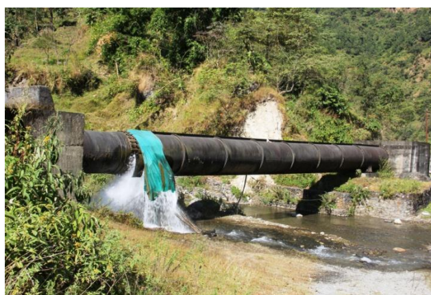
Leakage in Penstock Pipe in Khudi HEP
